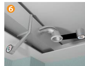
On ventilating ducts
